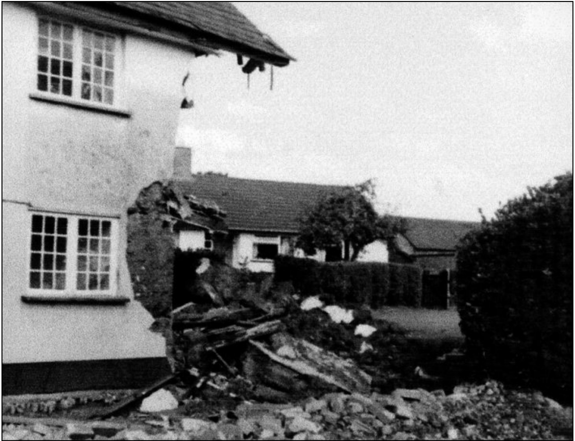
An adjacent cottage was also badly damaged
