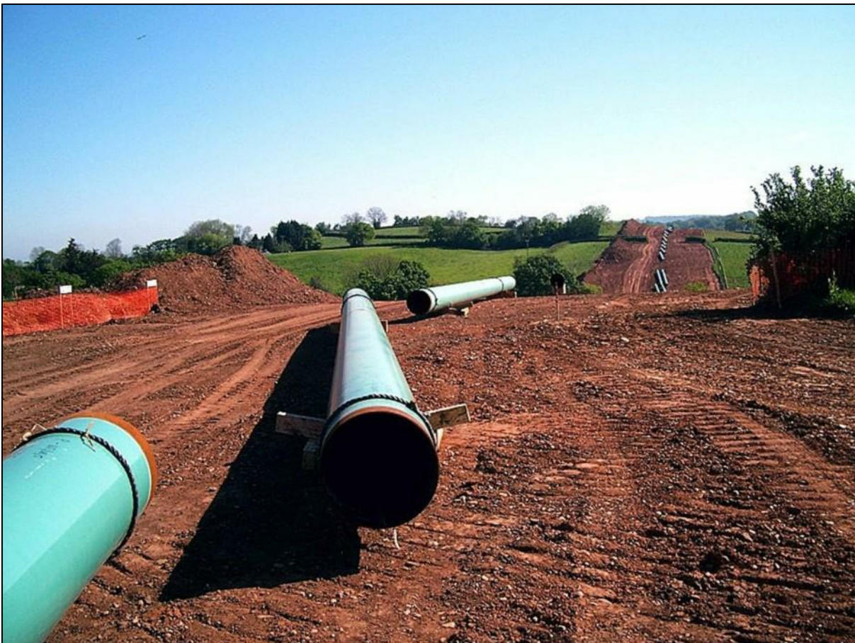
High pressure gas pipeline going through Woodbury Parish 2007.
